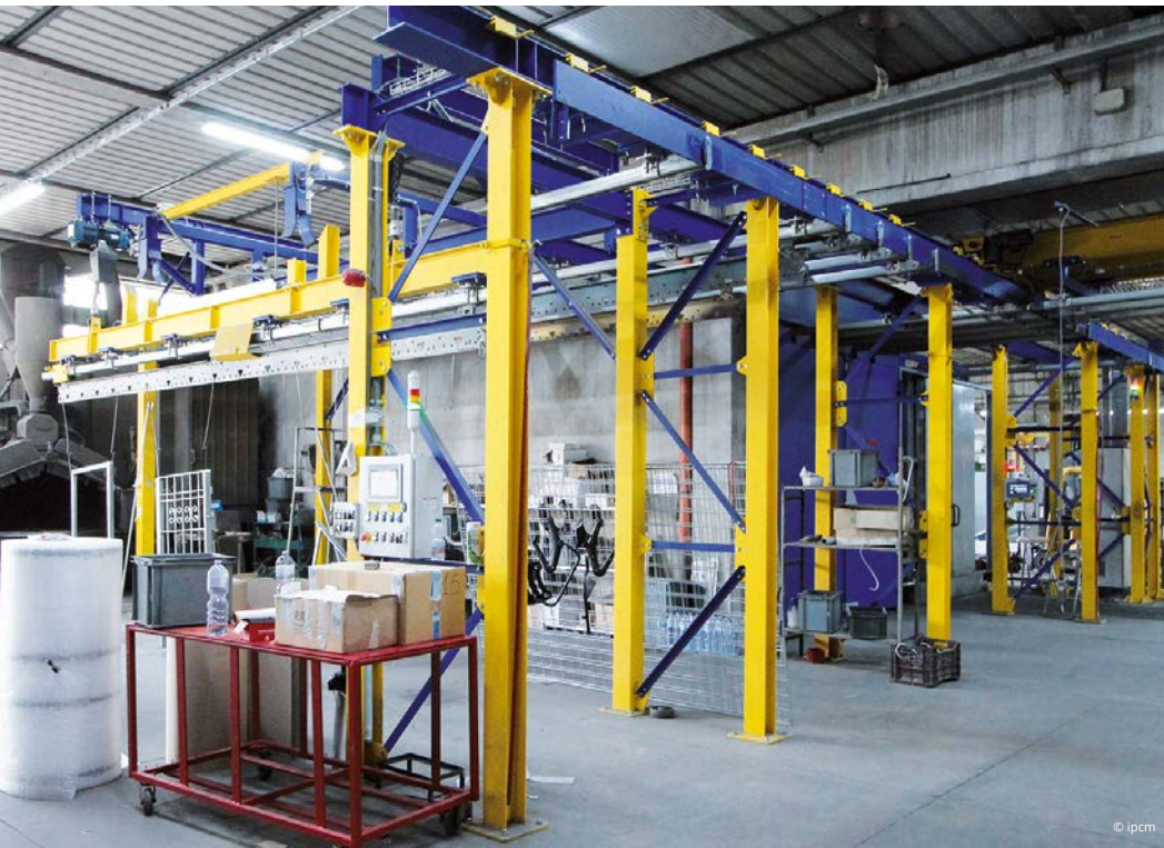
The loading/unloading station.
